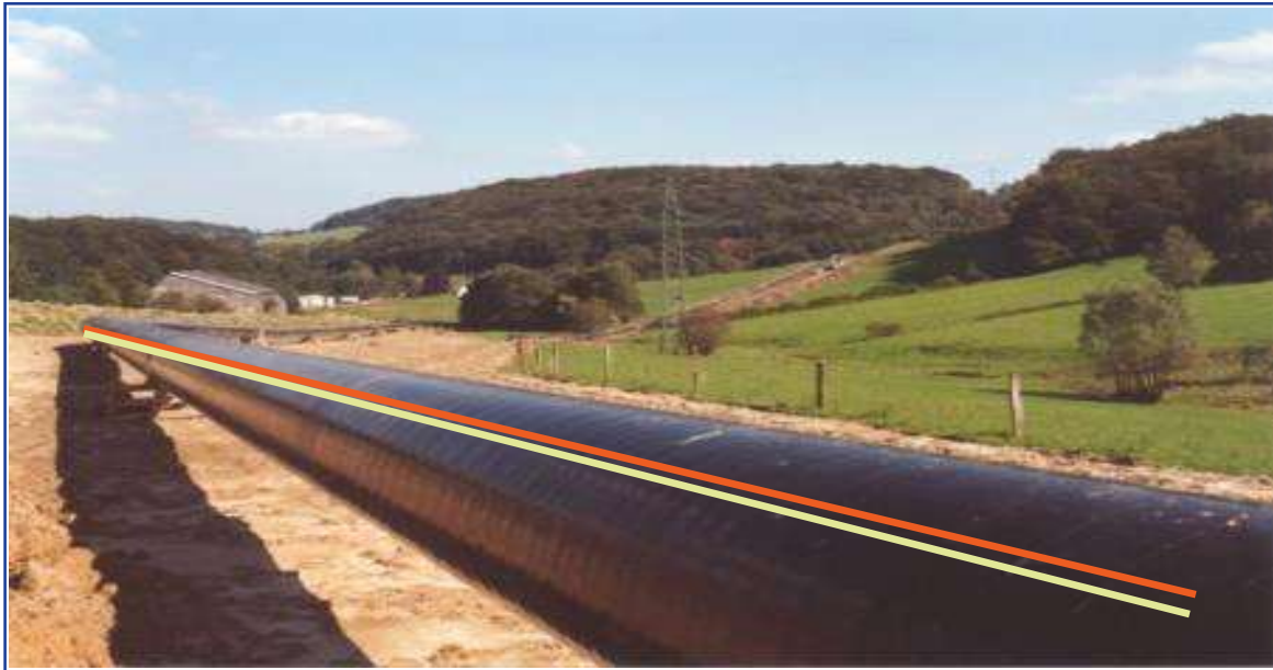
Fig. 3. Loosed optical cable and tight-buffer optical cable were connected together and installed on the pipe.
