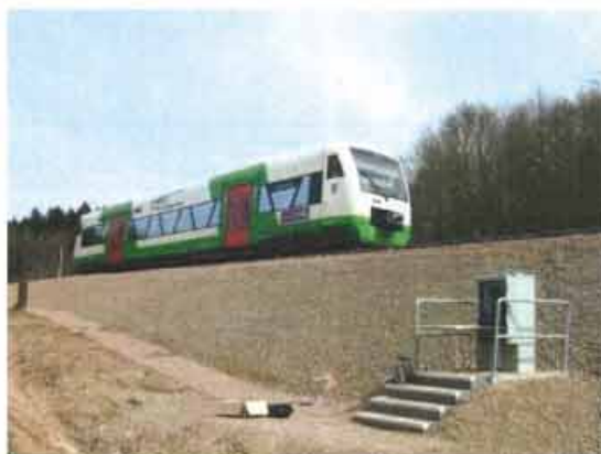
Fig.2 Outdoor housing of the measuring units
